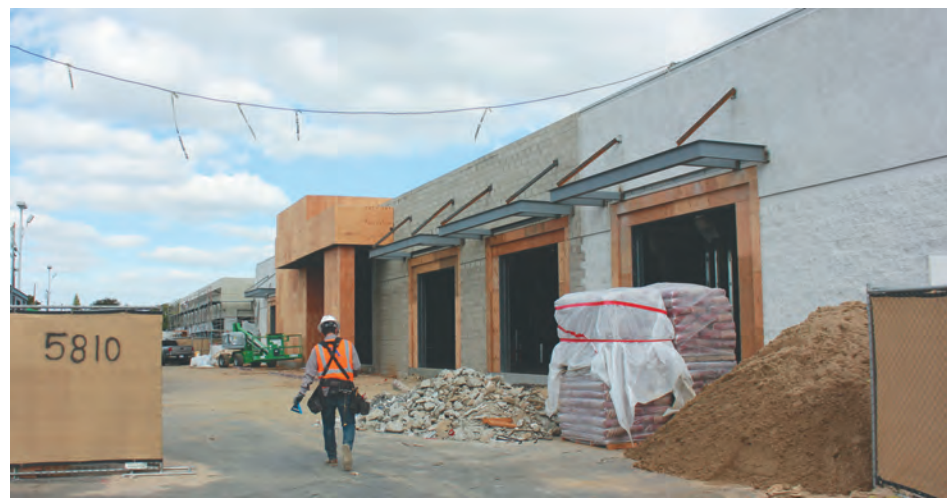
A complete interior and exterior remodel of the 35,000-square-foot L.A. Fitness gym is underway at the South & Downey Shopping Plaza in North Long Beach. (Photograph by the Business Journal's Brandon Richardson)
