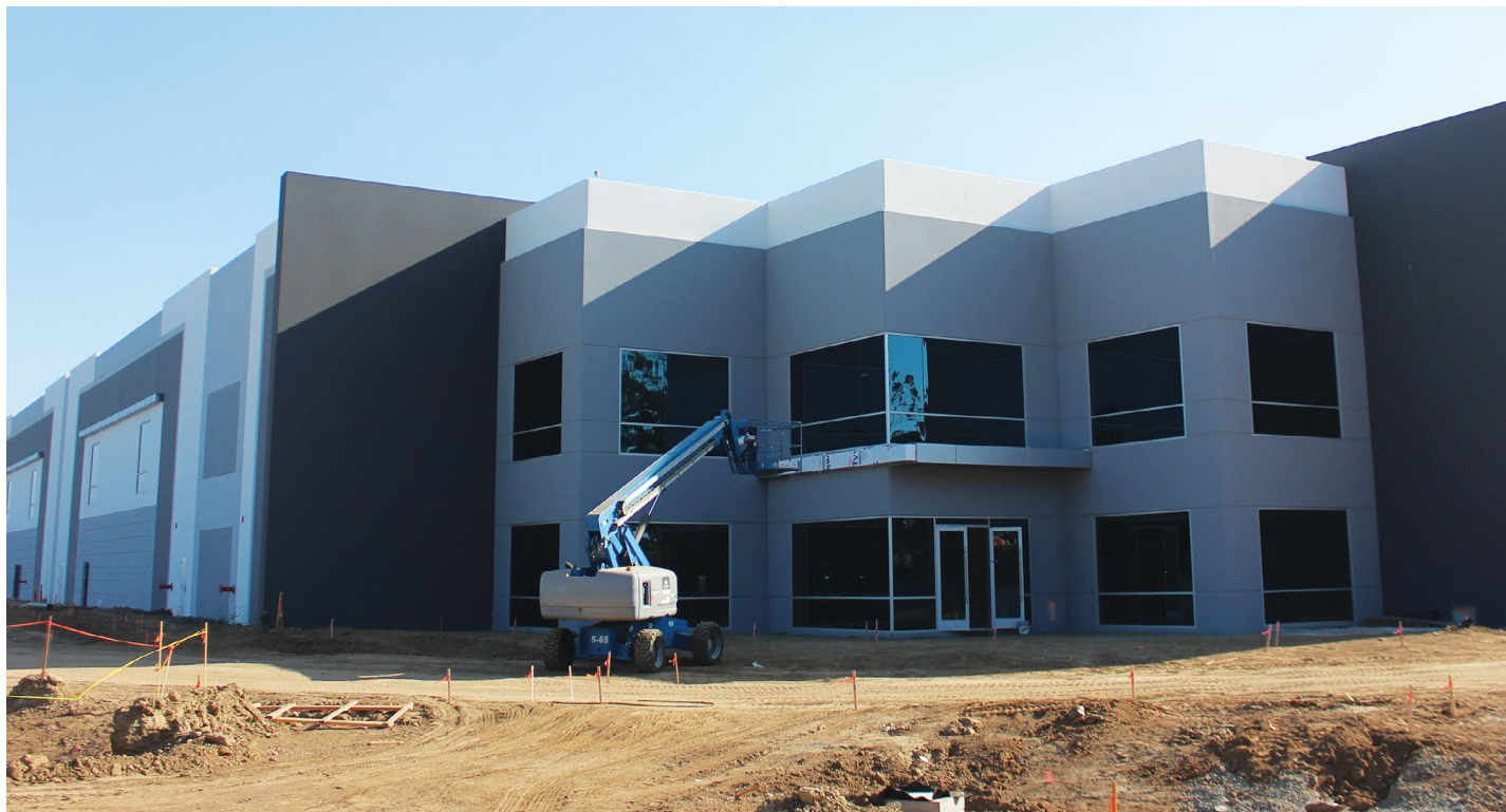
Exterior finishes are underway at Pacific Pointe Northwest, the final major development at Douglas Park by Sares-Regis Group. With four buildings totaling approximately 390,000 square feet, construction is expected to be fully complete by October. The first building is slated for completion this month. (Photograph by Brandon Richardson.)
